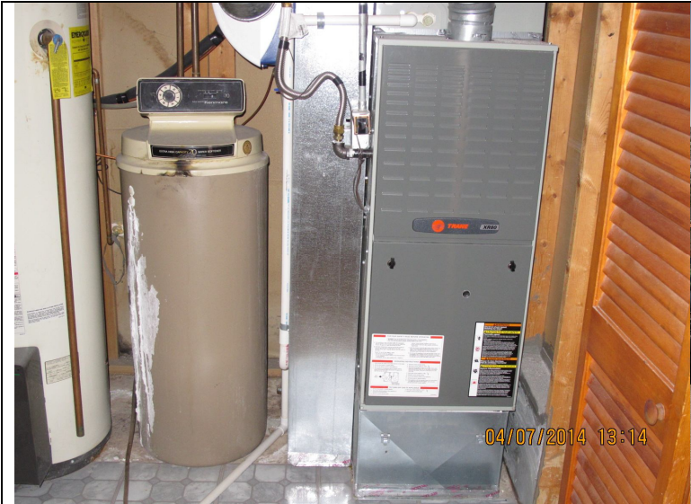
Furnace & Water Heater in Lower Level
